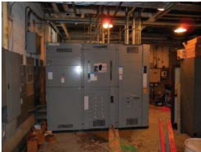
New Electrical Panel
