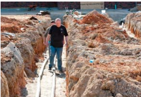
Well Field Piping which is a continuous loop from the building, through the well field, and back to the building.
