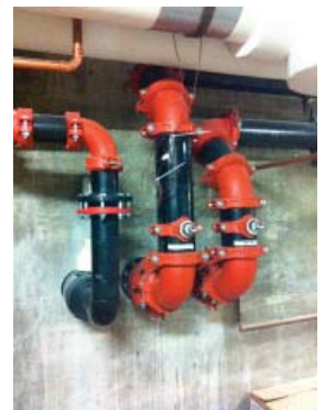
Geothermal loop piping showing out/in water lines
