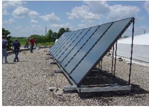
Well Field After Completion and Solar Collectors for Domestic Hot Water
